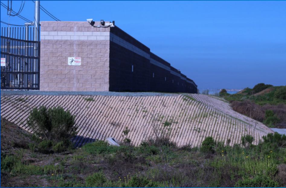
SDG&E's Bay Boulevard substation was built on a platform to raise it farther above sea level.
